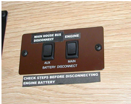
Disconnect panel (over the entrance door)
